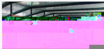
5. Sodium hypochlorite generator equipment
